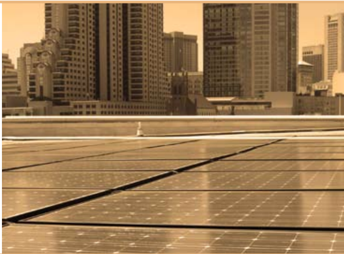
A 675-kilowatt flat roof solar PV system on the Moscone Convention Center in San Francisco, California.
