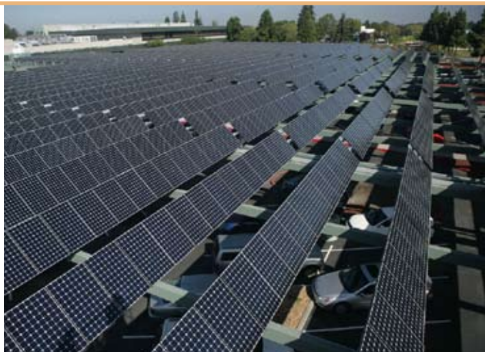
A 2-megawatt solar PV system, one of the largest corporate solar power installations in the U.S., covers the Applied Materials parking lot in Sunnyvale, California. The 8,000 panels change their tilt to track the sun’s position.
