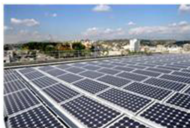
A commercial rooftop solar project.
