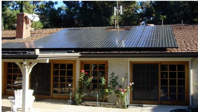
A 7 kilo-watt residential solar system
